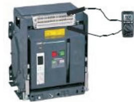
Figure 56. Inspection of secondary circuit
